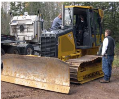
Club members at the end of the day working on the Fish Lake re-route. These photos were provided from Greg McDonald.
